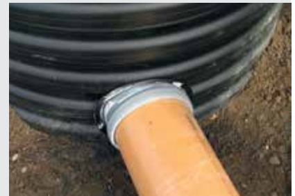
6. The "in-situ" insert is now ready for a sewer pipe to be inserted.
