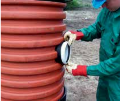
4. If installation is difficult, the edges of the hole can be coated with lubricant.
