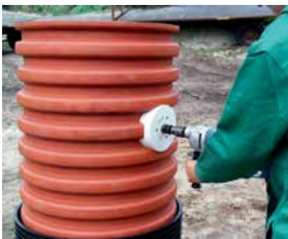
1. A hole is made in the corrugated pipe with a special jigsaw.
