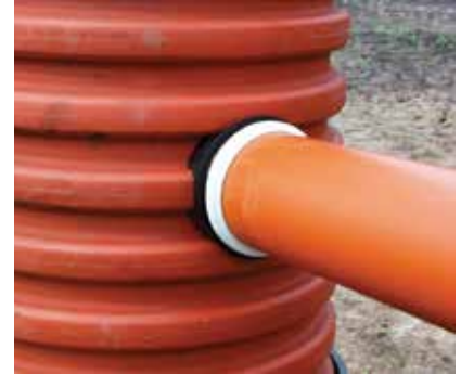
6. The "in-situ" insert is now ready for a sewer pipe to be inserted.
