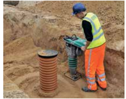
12. The excavation must be filled with layers of max. 30 cm thickness, burying the chamber evenly from each side up to the height where the chamber top will be placed.
