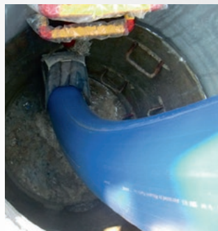
Japan, Osaka, DN250, Potable Water
