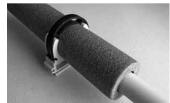
For hot water, the clip must be one size larger than the pipe (needs to be fitted over the insulation).
