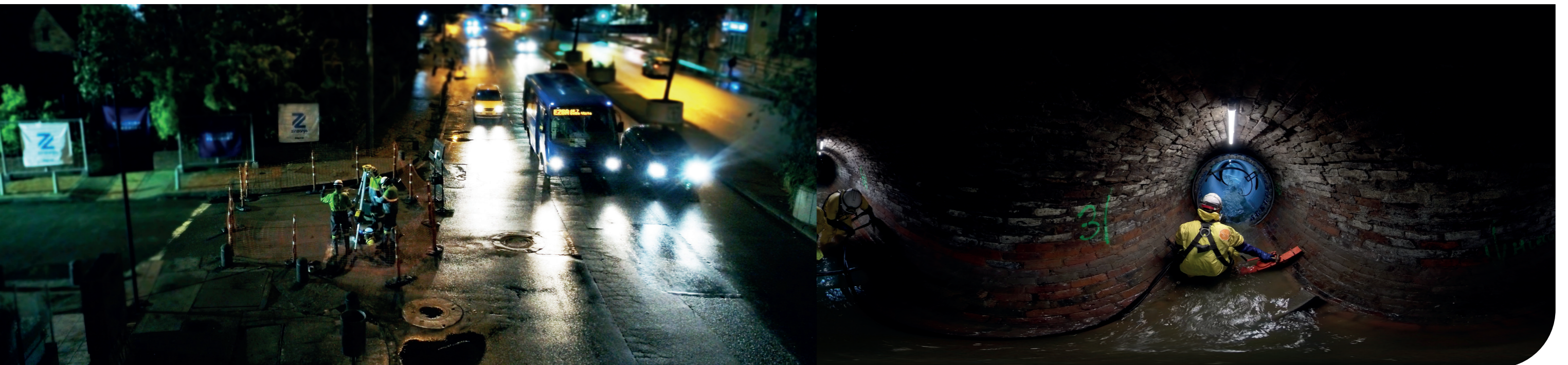
Working on the Bogotá sewage system with minimal inconvenience to local residents and traffic. Bogotá, Colombia.
