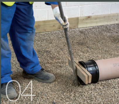
04 Larger pipe sizes can be jointed with the assistance of a bar
