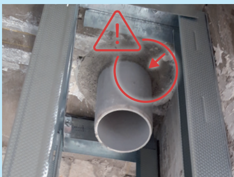
Figure 20: Forgotten structure-borne sound decoupling
