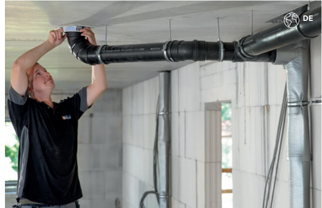
Figure 39: Wastewater pipe with sound insulation hose
