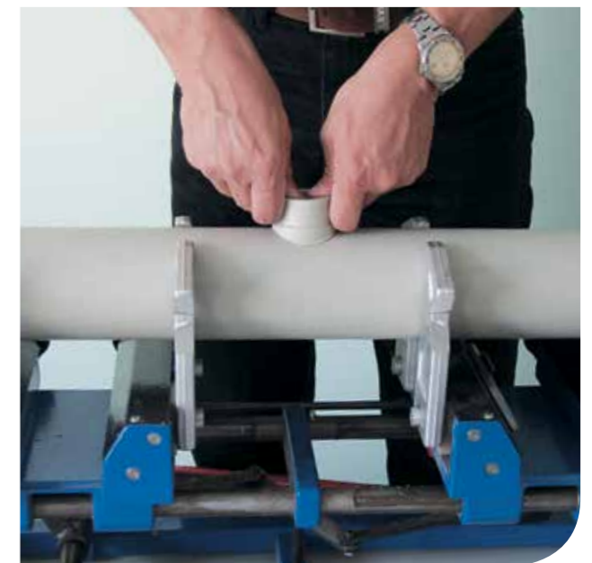
4. Put the heated saddle on the heated hole and fasten for about 16 seconds. You can fill the pipe with water and expose it to pressure one hour later.
